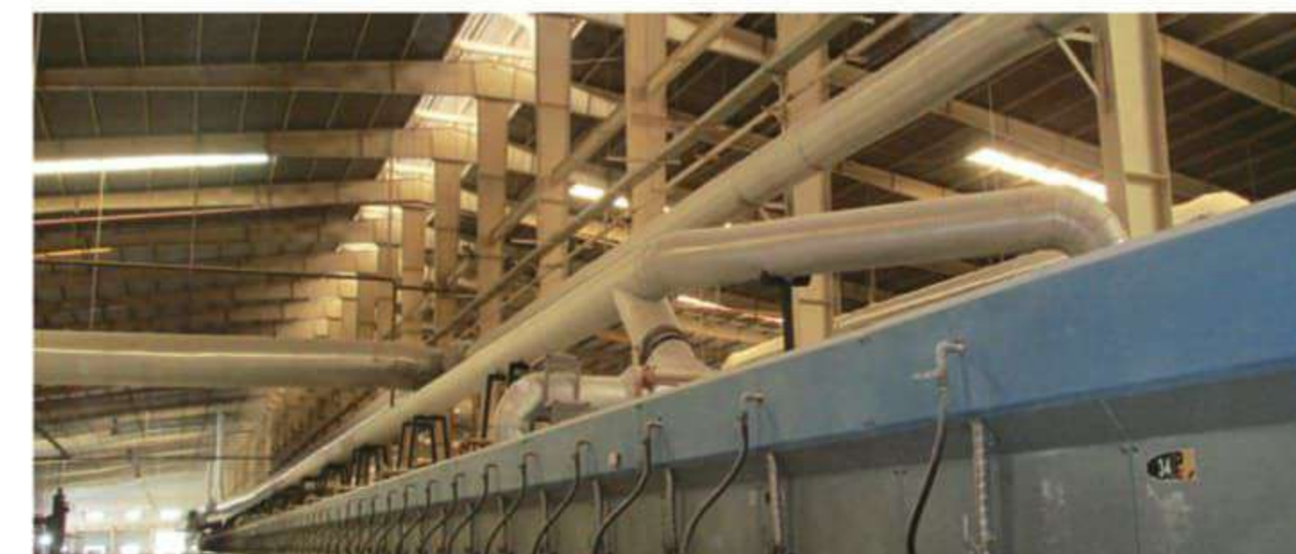
Dust Collection and Raw Material Recycle System / 中央集塵系統
